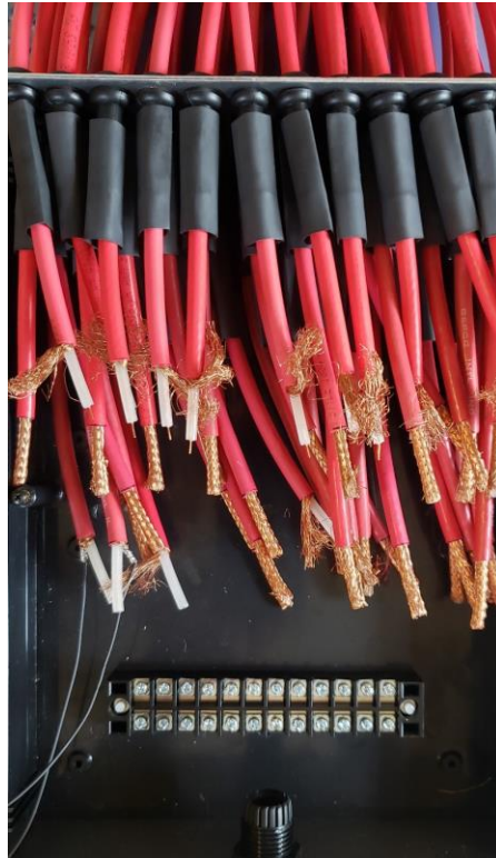
Stripped jackets of SHV cables, terminal block, and cable strain relief for Radiall-to-SHV adapter
